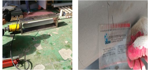
Fig. 7 Photos for jacking and crack width measurement
